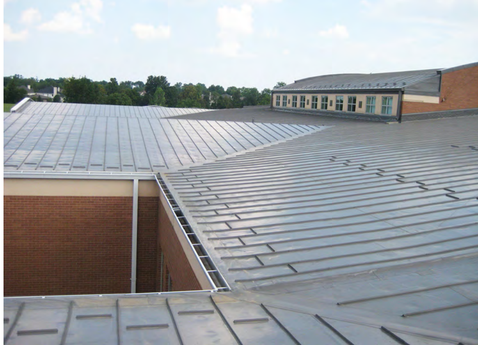
The flexibility inherent in the Décor Roof System made the job of Midland Engineering, the roofing contractor, easier when faced with the many flashing details, elevation changes, valleys and roof configurations at the Smoky Row School.
